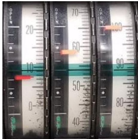
Figure 10. Current control room “green band indication.”
