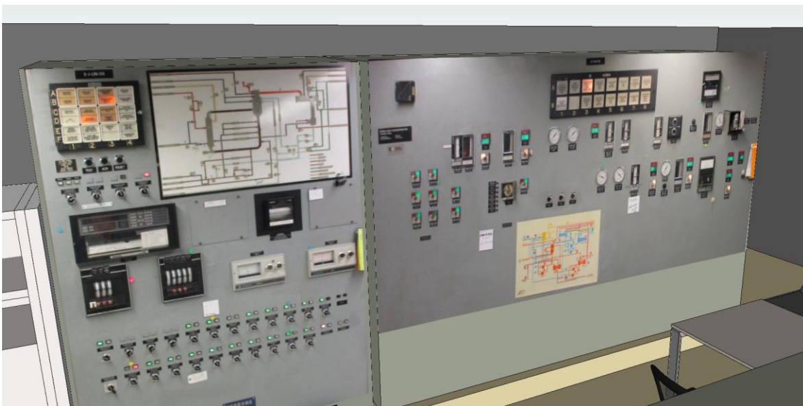
Figure 16. 3-D model of the evaporator panel and BAC panel in existing radiological waste control room.
