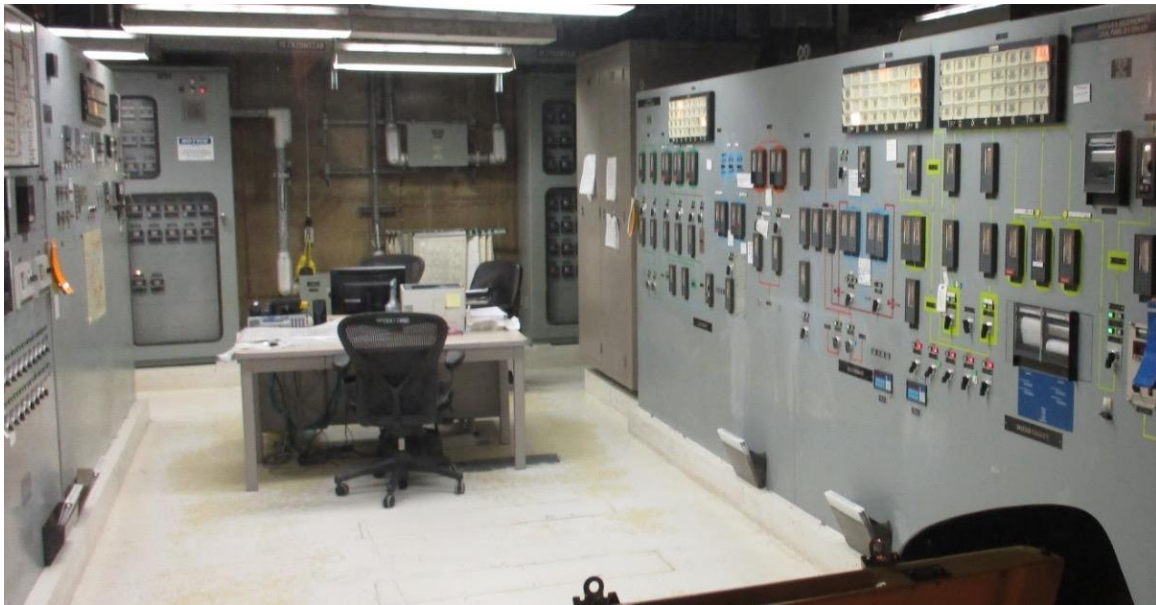
Figure 12. The actual radiological waste control room.
