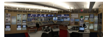
Leverage Glasstop Simulator for I&C Design, Procedure Development in Addition to Operator Training
