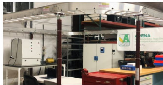
Fig. 1 ARENA Cable Test Bed
