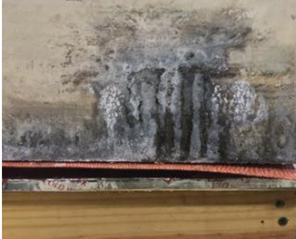
Figure 7. Damage location 1 – cracking and powder effluence.
