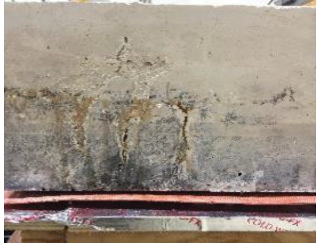
Figure 8. Damage location 2 – clear gel effluence.
