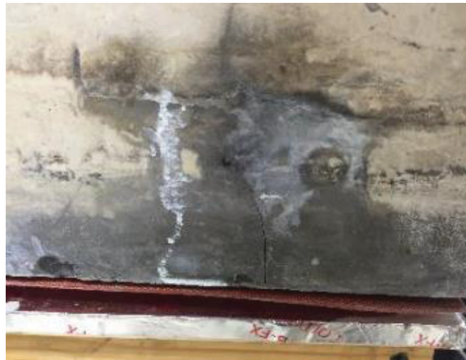
Figure 9. Damage location 3 – cracking and powder effluence.
