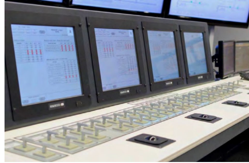
Example Safety Display Installation
