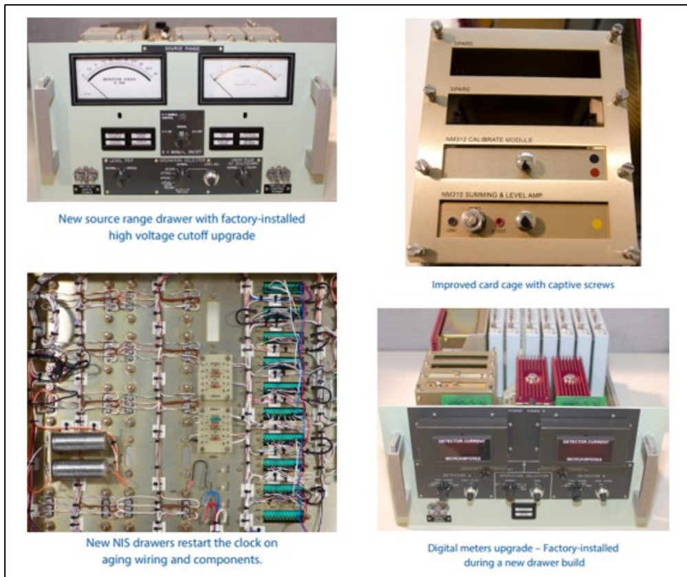
Figure 2-1. Upgraded Nuclear Instrumentation Protection Equipment Examples
