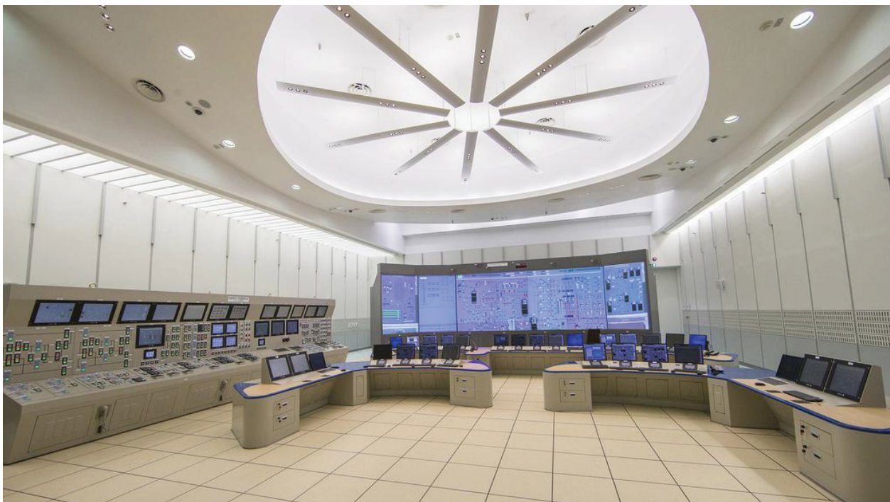
Figure 5. Simulator for the Main Control Room of the APR-1400 at Barakah, UAE
