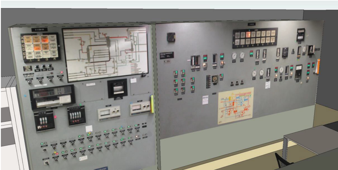
Figure 25. 3-D model of the evaporator panel and BAC panel in existing radiological waste control room.
