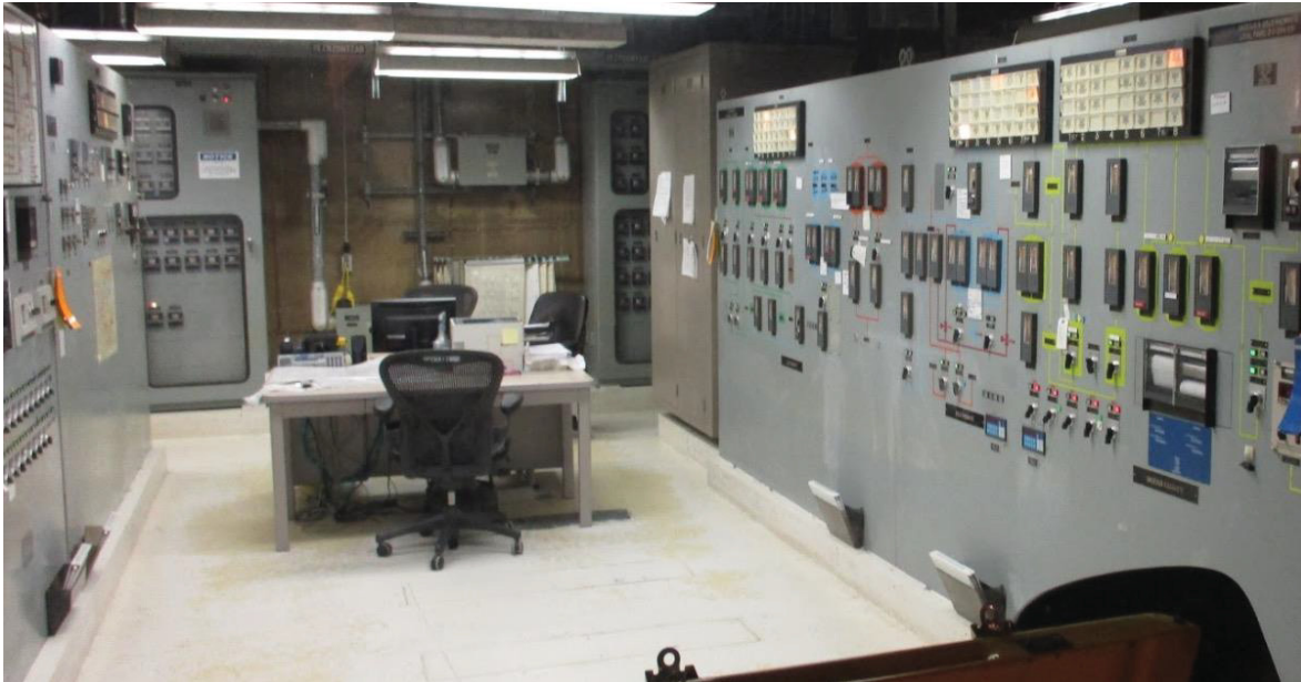
Figure 21. The actual radiological waste control room.
