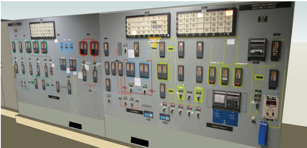
Figure 24. 3-D model of the LRS panel and gaseous and solid radiological waste panel in existing radiological waste control room.
