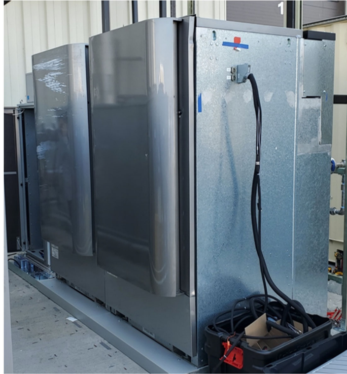
Figure 7. Low pressure 100 kW HTE subcomponent module installed at INL.
