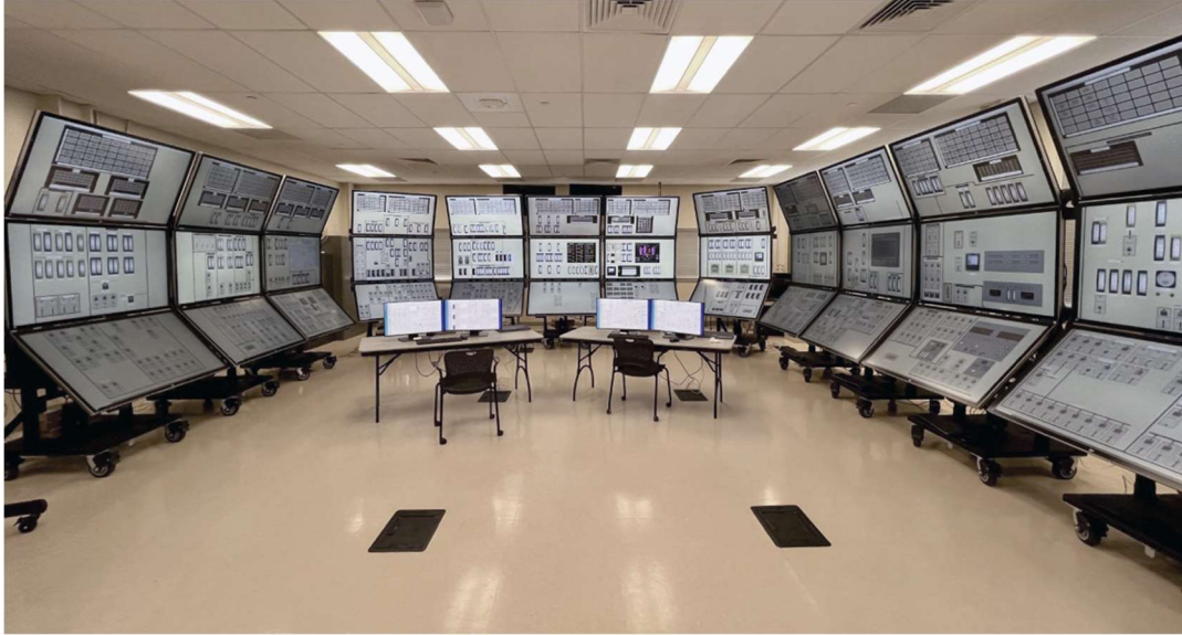
Figure 1. Human Systems Simulation Laboratory showing the GSE GPWR analog control room panels represented virtually on touch screen displays.
