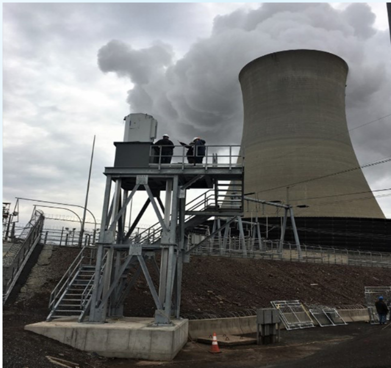
Figure 3. A remotely operated "Single Sentry-II" installation, replacing a guard post. ROWS Configuration.
