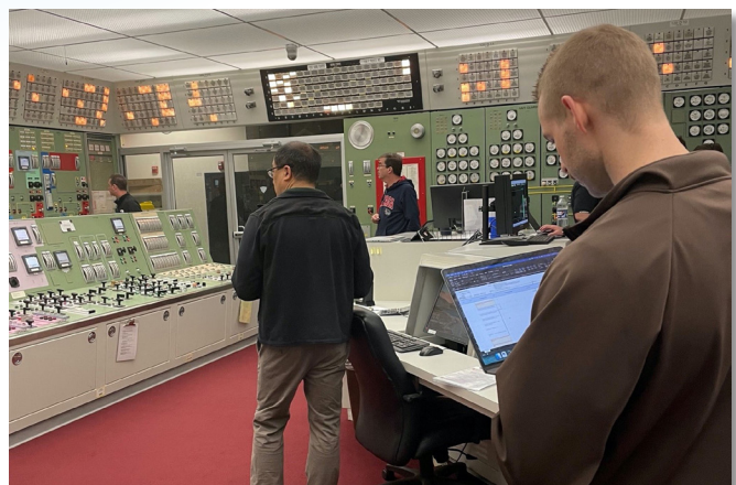
INL Human Factors Engineers Assessing Limerick Generating Station Main Control Room Operations to Support Design Changes
