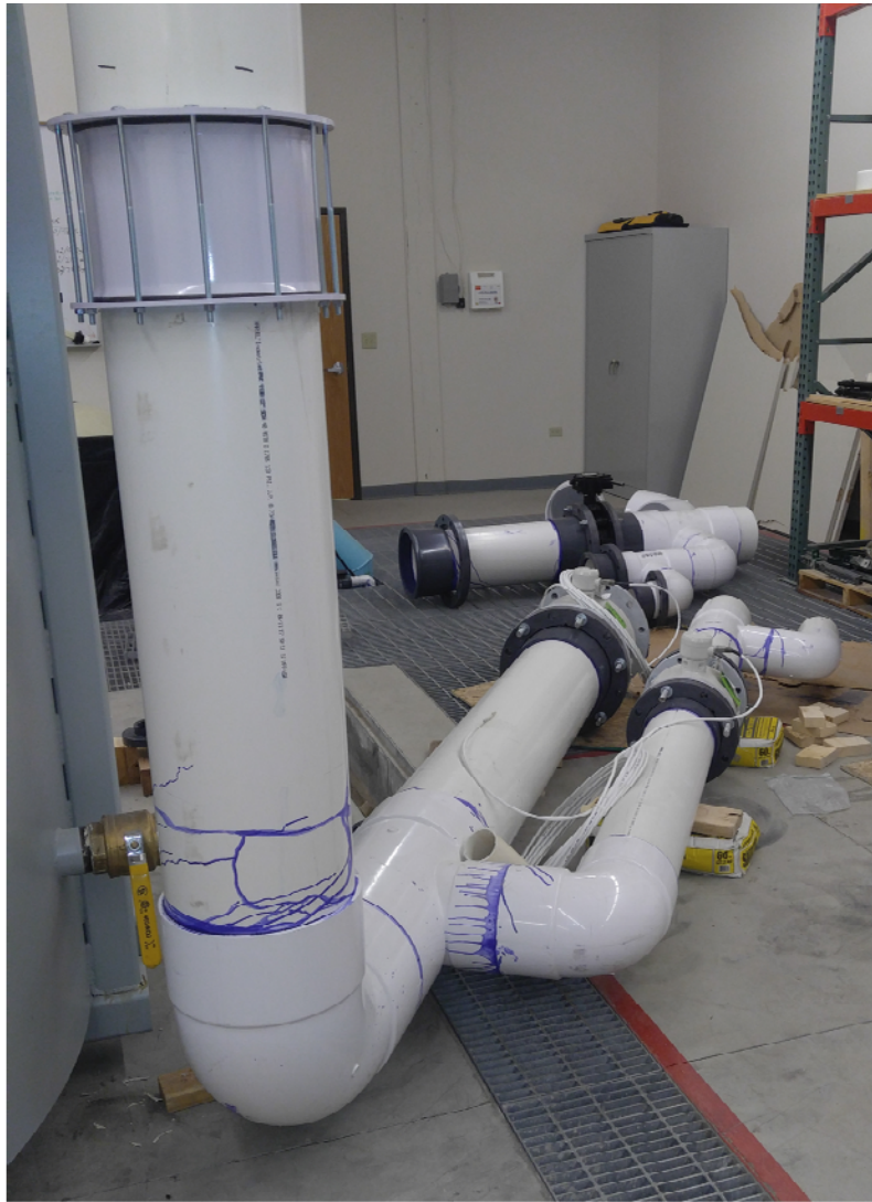
Figure 11. PET downstream piping bifurcations, flow meters, and control valves.
