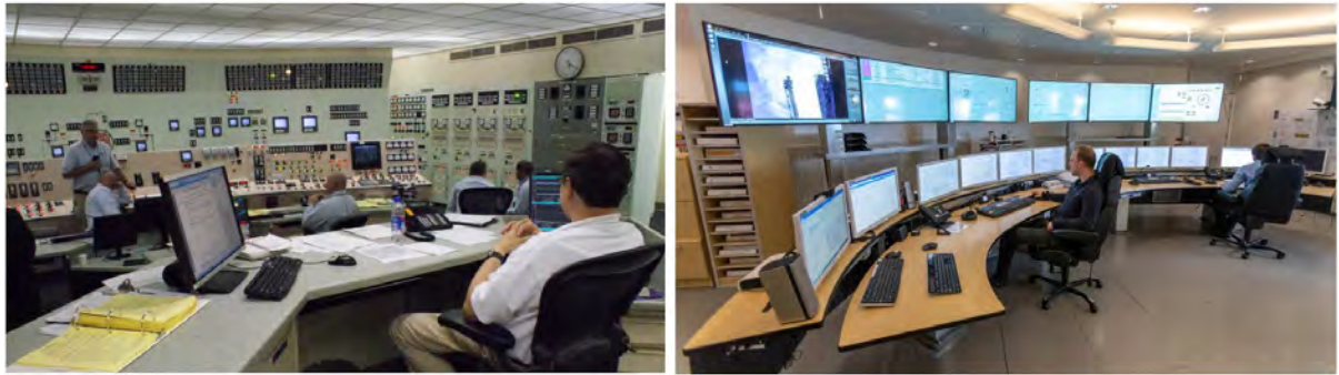
Figure 7. Illustration of a typical U.S. nuclear plant control room (left) and a modern petroleum control room (right).
