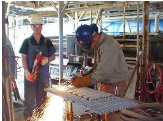
Figure 1. Fire watch for welding hot work performed in an industrial environment (U.S. Department of Labor 2019).
