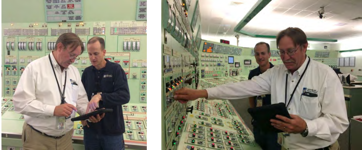
Figure 5. A control-room operator and a field operator validate the CBP system.
