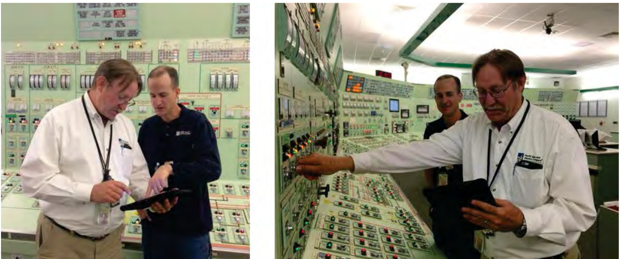
Figure 2. A DCPP control-room operator and a field worker validate the CBP system.
