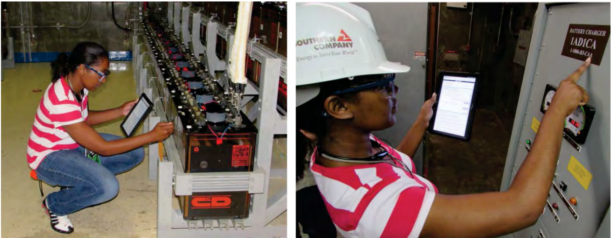
Figure 3. A maintenance technician at Plant Vogtle performs the battery and charger test and inspection work order.
