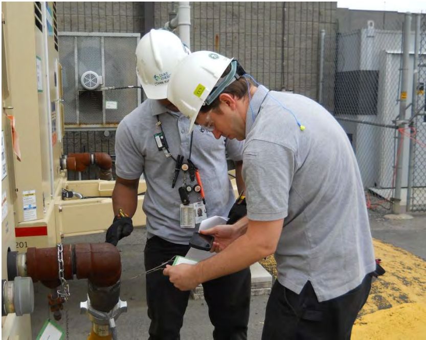
Figure 5. Two AOs at Catawba Conducts a Walkdown of The CBP at The Actual Job Site During The Pre-Validation Activity.
