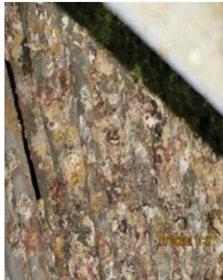
Figure 7.23. Bird feces on cables in trays.
