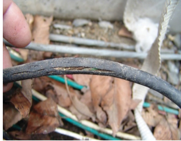
Figure 7.3. Cracked butyl jacket. Photo courtesy of EPRI.
