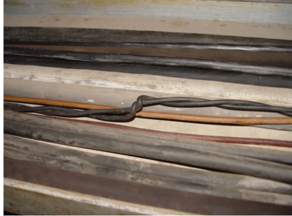
Figure 7.9. Kinked conductors. Photo courtesy of EPRI.
