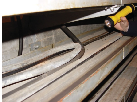
Figure 7.5. Severely bent cable. Photo courtesy of EPRI.
