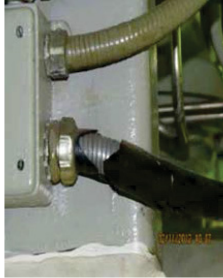
Figure 7.21. Ripped seal-tight on conduit on RCB chiller.
