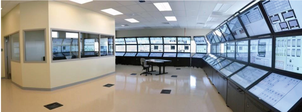
Figure 1. Department of Energy's Human System Simulation Laboratory reconfigurable simulator for conventional control rooms.
