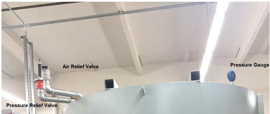
Figure 5. PET reliefs and pressure gauge.
