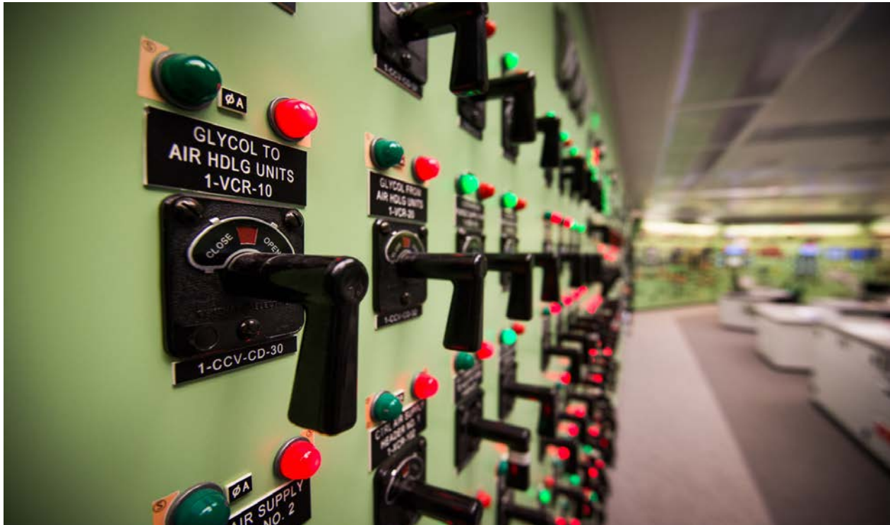
Figure 1 Example of analog control board found in many of the US Nuclear industry
