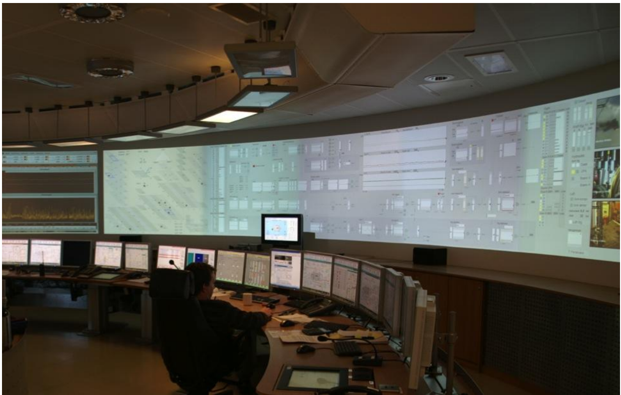
Figure 6. Large Screen Display from Snorre A Offshore Oil Platform.
