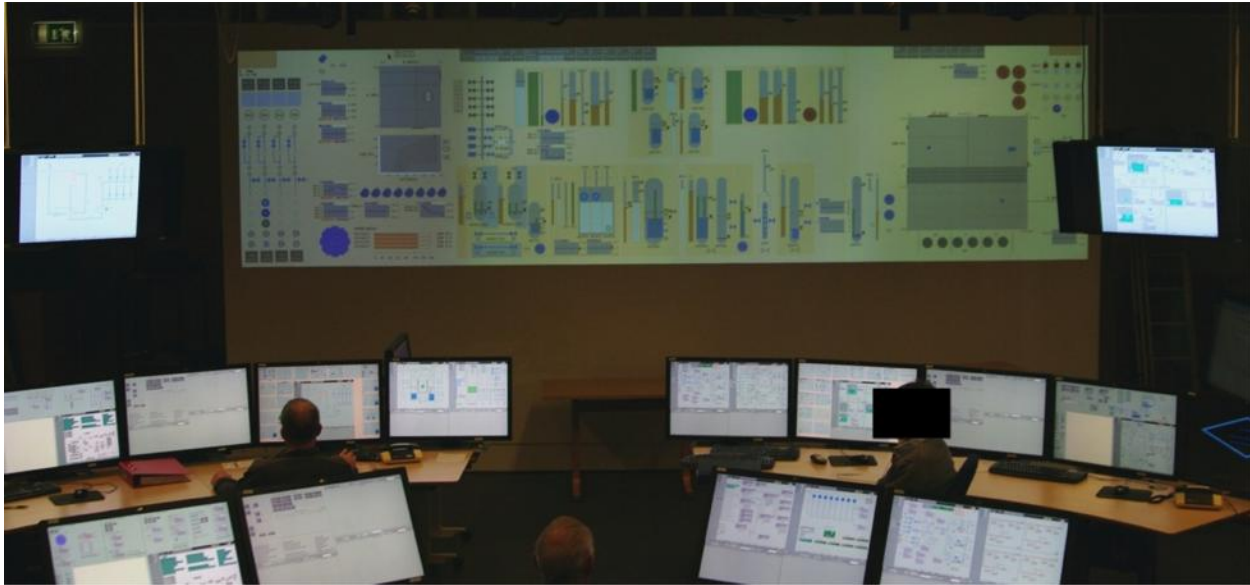
Figure 2. A Fully Digital Control Room for a Nuclear Power Plant at OECD Halden Reactor Project.
