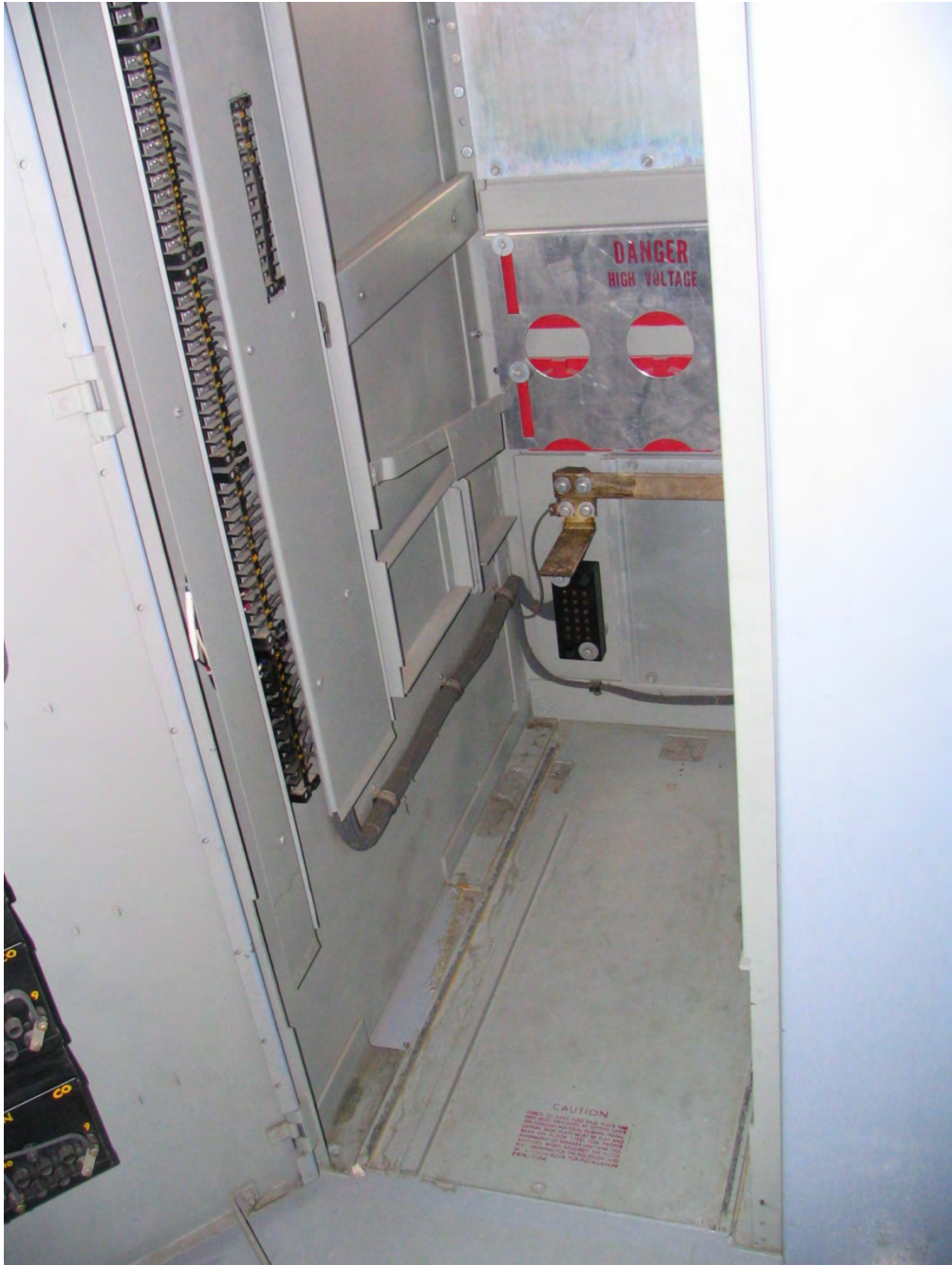
Figure 3-13 – Medium Voltage Switchgear 670-E-2
