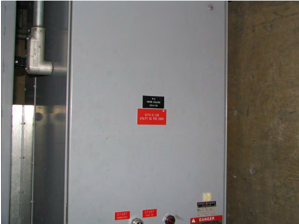
Figure 3-12 – Low Voltage Switchgear 670-E-28
