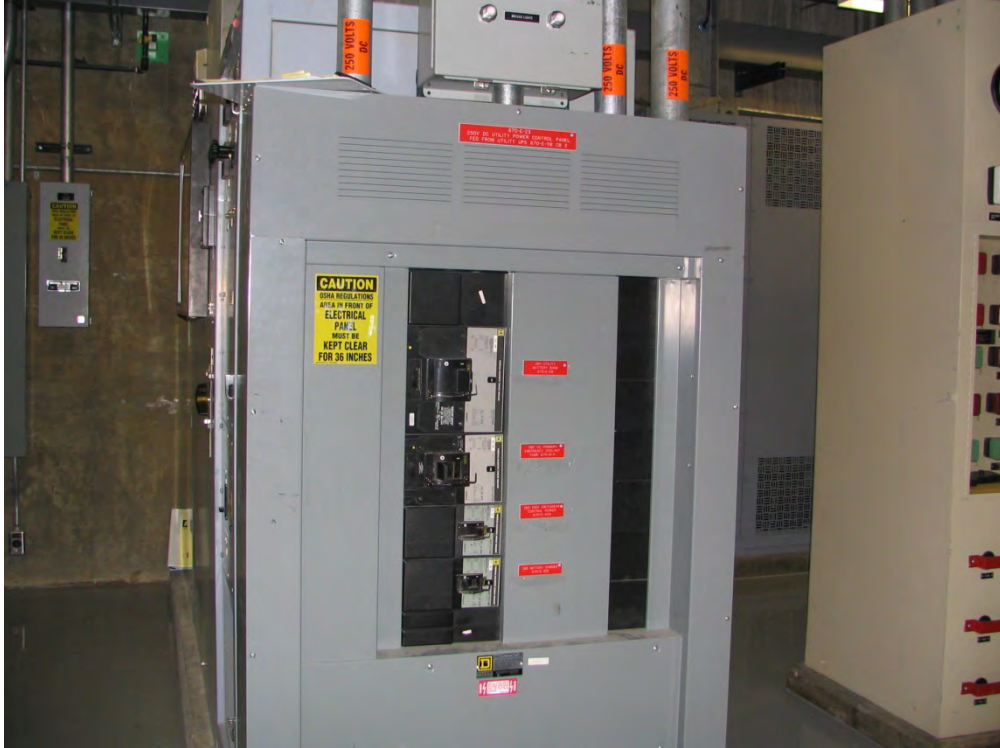
Figure 3-11 – Distribution Panel 670-E-23
