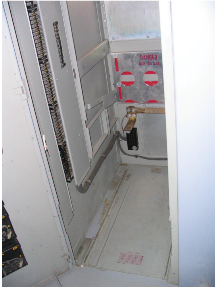
Figure 2-10: Medium voltage switchgear 670-E-2
