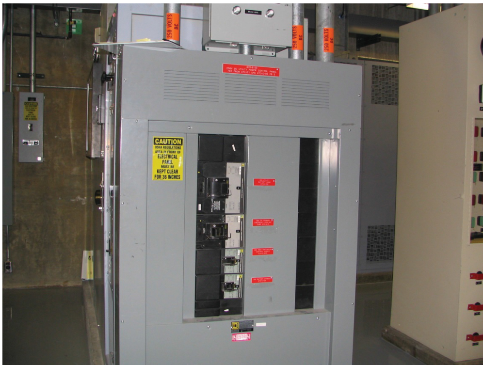
Figure 2-9: Distribution panel 670-E-23
