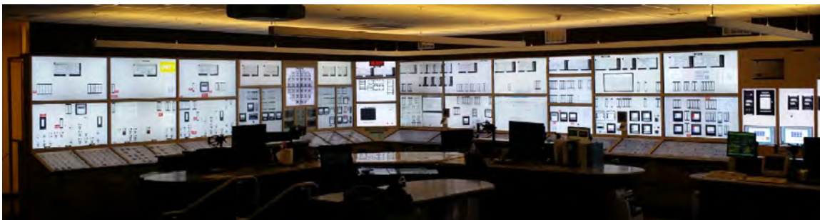
Figure 9. Representative utility nuclear plant glasstop main control room simulator.
