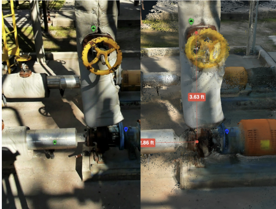
Figure 2. Side-by-side comparison of photogrammetry and LiDAR data collected with mobile mapping, including measurements in the Ei viewer.
