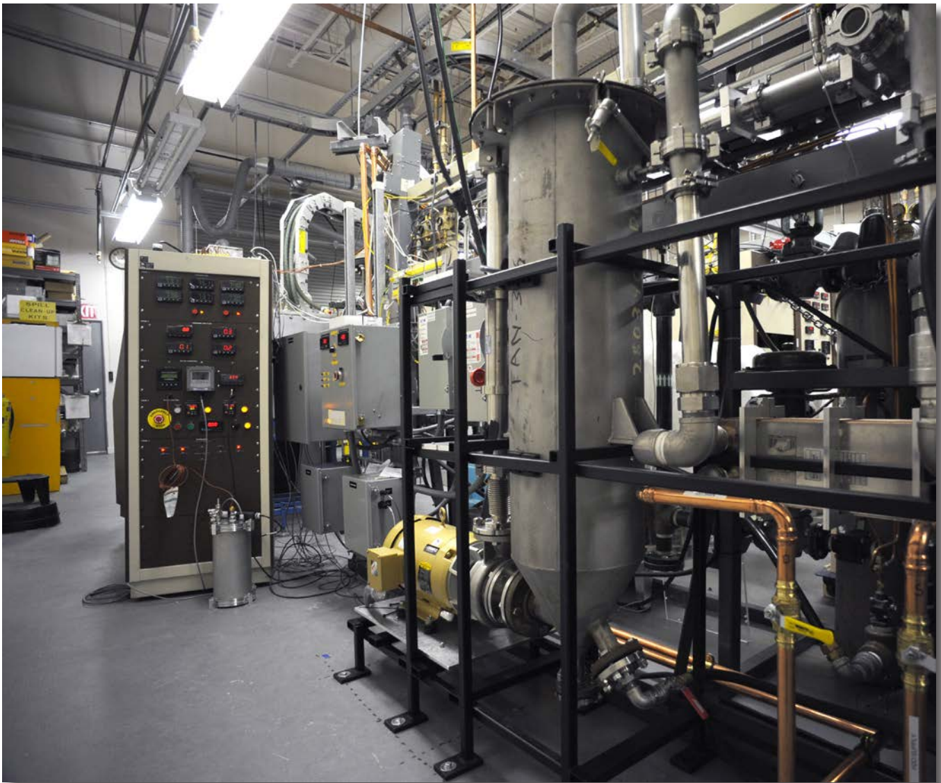
Figure 7. Photo of the assembled hot water corrosion flow test equipment.
