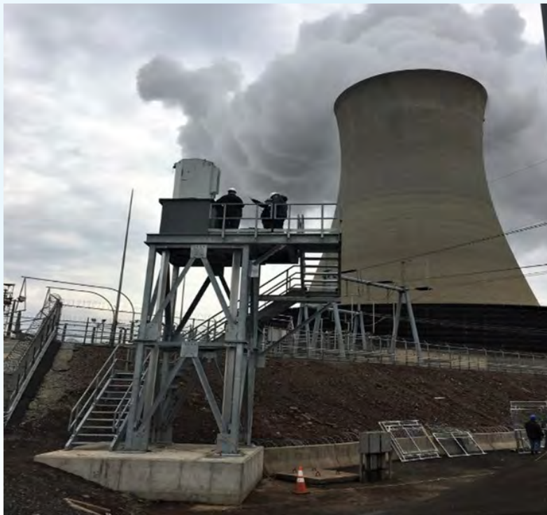
Figure 3. A remotely operated "Single Sentry-II" installation, replacing a guard post. ROWS Configuration.
