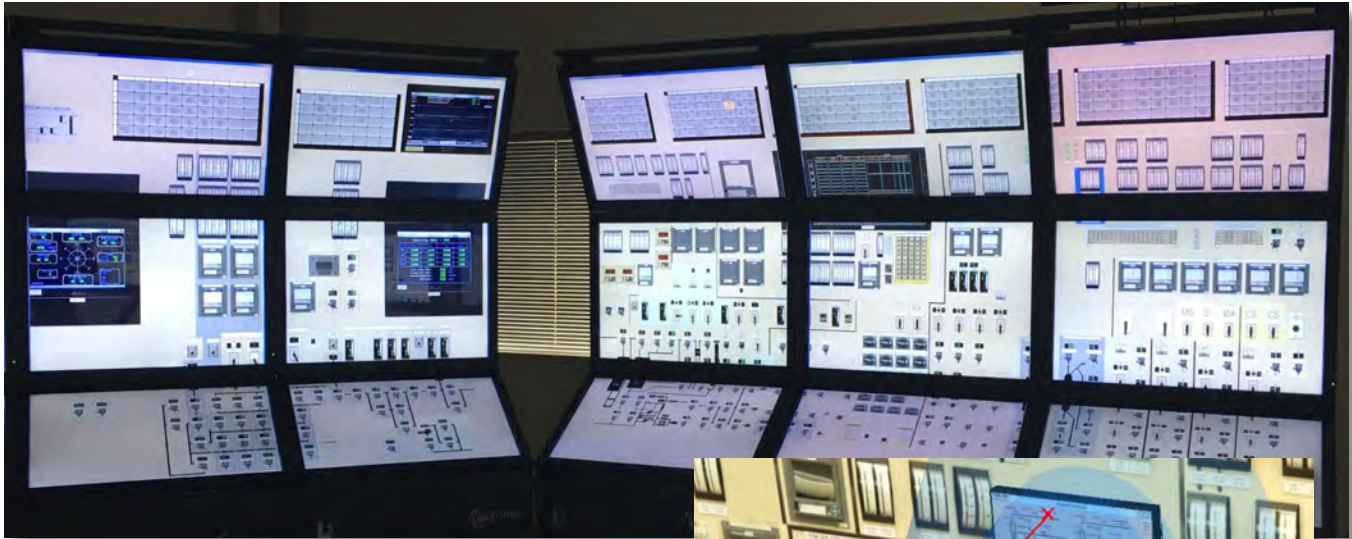
Figure 5. LWRS Program's Human Systems Simulation Laboratory (at Idaho National Laboratory) configured as the Braidwood main control room so the effect of upgraded digital I&C on operator and overall system performance can be evaluated (above).
