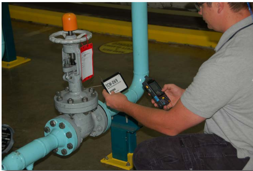
Figure 6. A Catawba Nuclear Station maintenance technician using wireless mobile worker technology to conduct valve maintenance.
