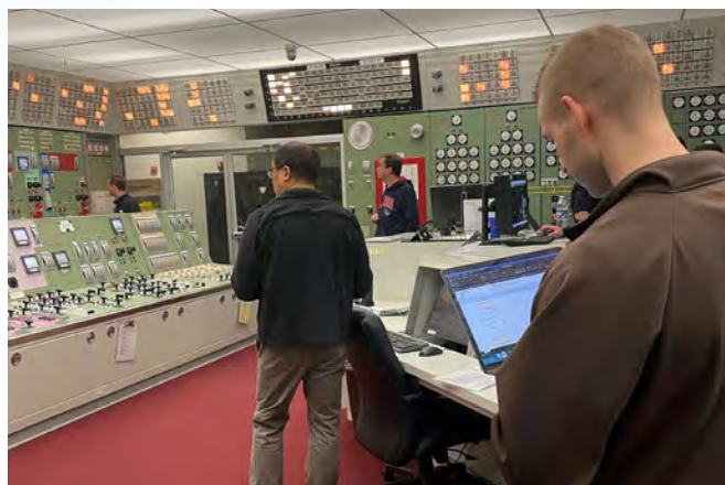
INL Human Factors Engineers Assessing Limerick Generating Station Main Control Room Operations to Support Design Changes
