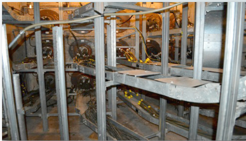
Figure 5. Zion Station Unit 2 cable penetration vault, outside containment.
