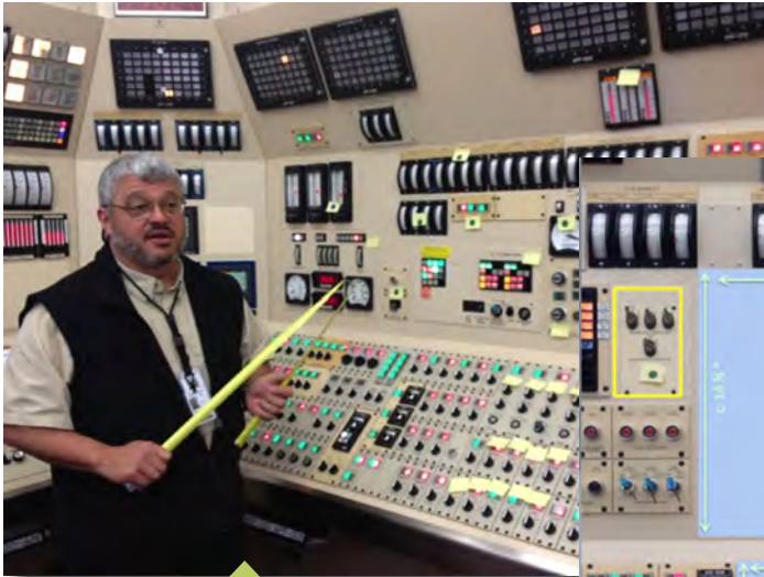
Figure 6. Matt Gibson of Duke Energy works with Advanced II&C Systems Technologies Pathway researchers to plan for the placement of new digital control system displays in an existing control room.
