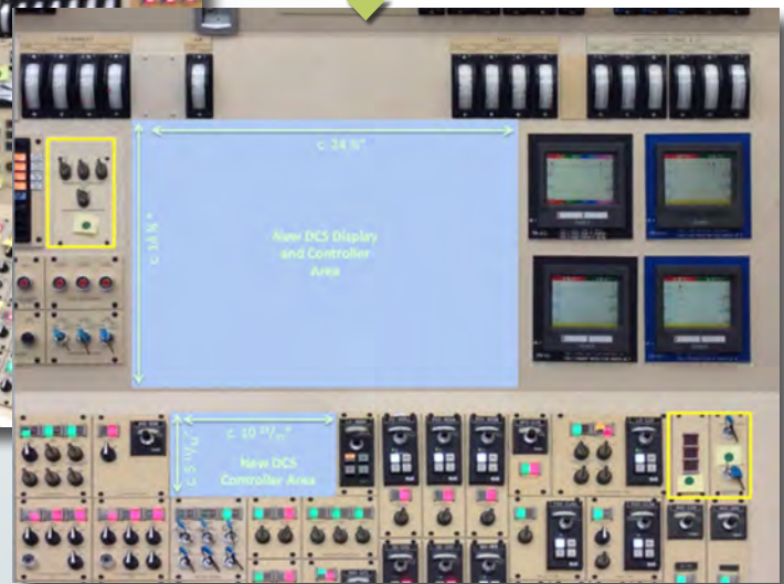
Figure 7. Example of modifications to the main control boards that enable the introduction of new digital displays.
