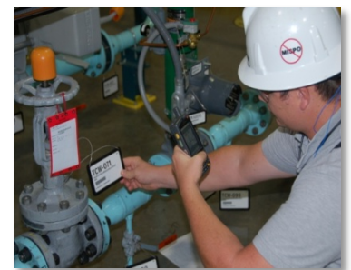
Figure 5 Operator at Catawba Nuclear Station using hand-held technology for component identification
