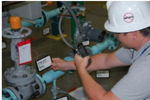
Figure 8 Operator at Catawba Nuclear Station using hand-held technology for component identification
