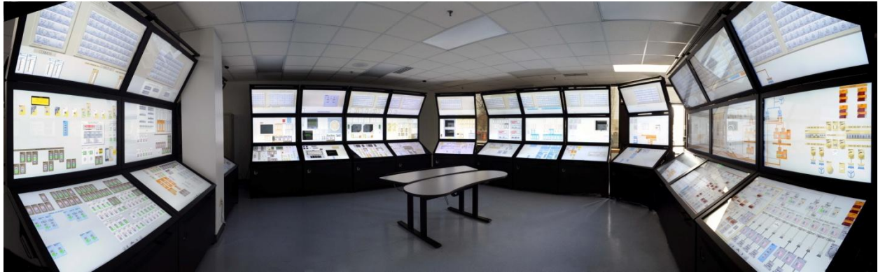
Figure 14 Human Systems Simulation Laboratory configured with bench-board style control bays for realistic simulation of current light water reactor control rooms
