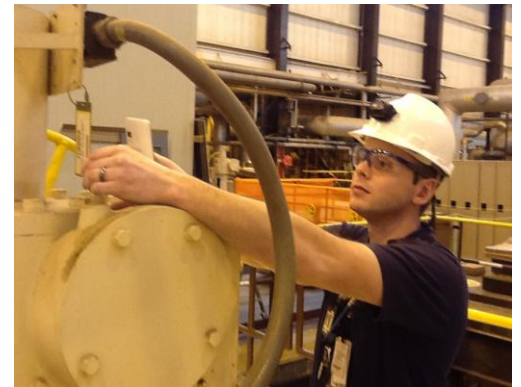
Figure 11 Operator uses hand-held technology to verify correct component identification at Byron Nuclear Station.
