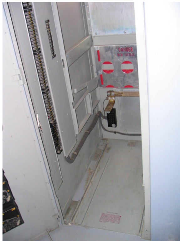
Figure 28. Photograph of medium voltage switchgear.
