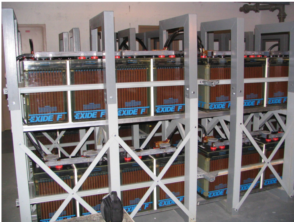
Figure 26. Photograph of battery rack.
