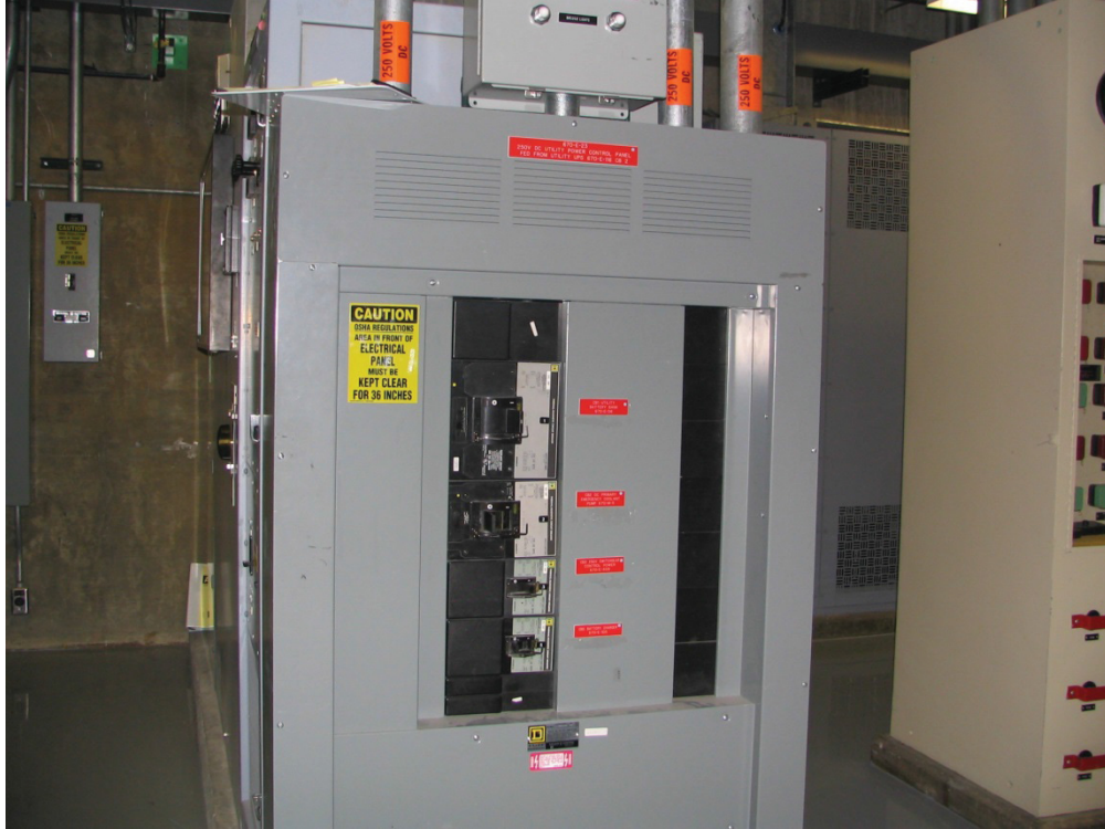
Figure 27. Photograph of distribution panel.
