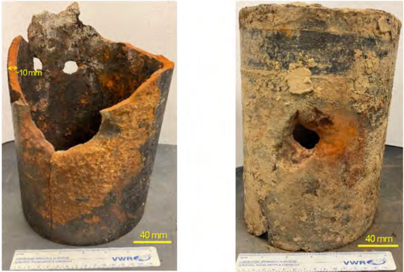
Figure 11. Failed cast iron pipes from ORNL water lines. [8]
