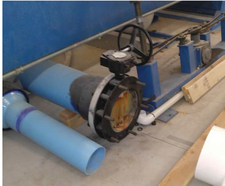
Figure 6. Existing 12-in pipe flanging.
