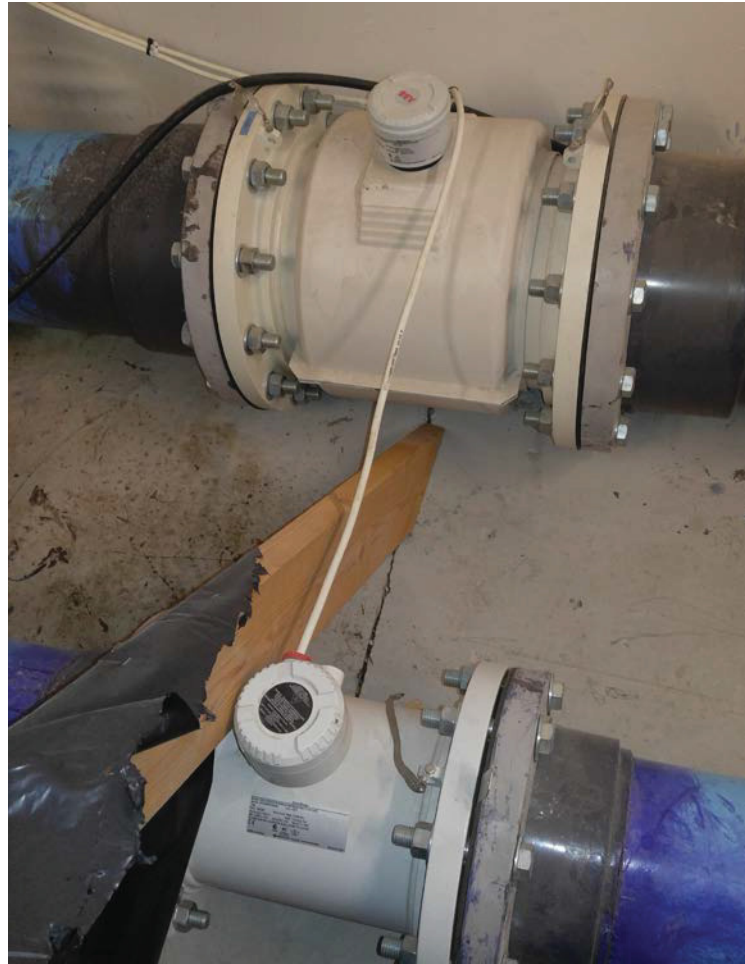
Figure 8. Existing 12 in flow meter (Top) and 8 in flow meter (Bottom).
