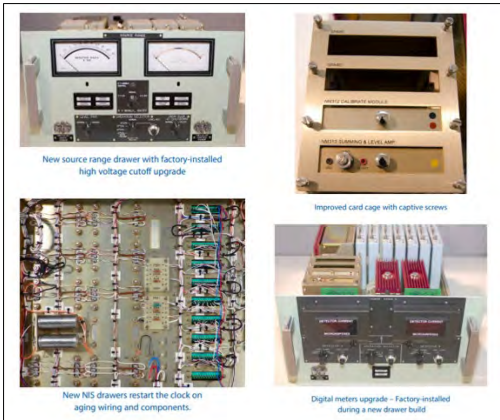
Figure 2-1. Upgraded Nuclear Instrumentation Protection Equipment Examples
