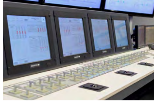
Example Safety Display Installation
