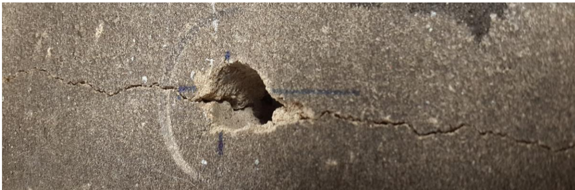
Figure 6. Crack produced by the freeze-thaw cycles.
