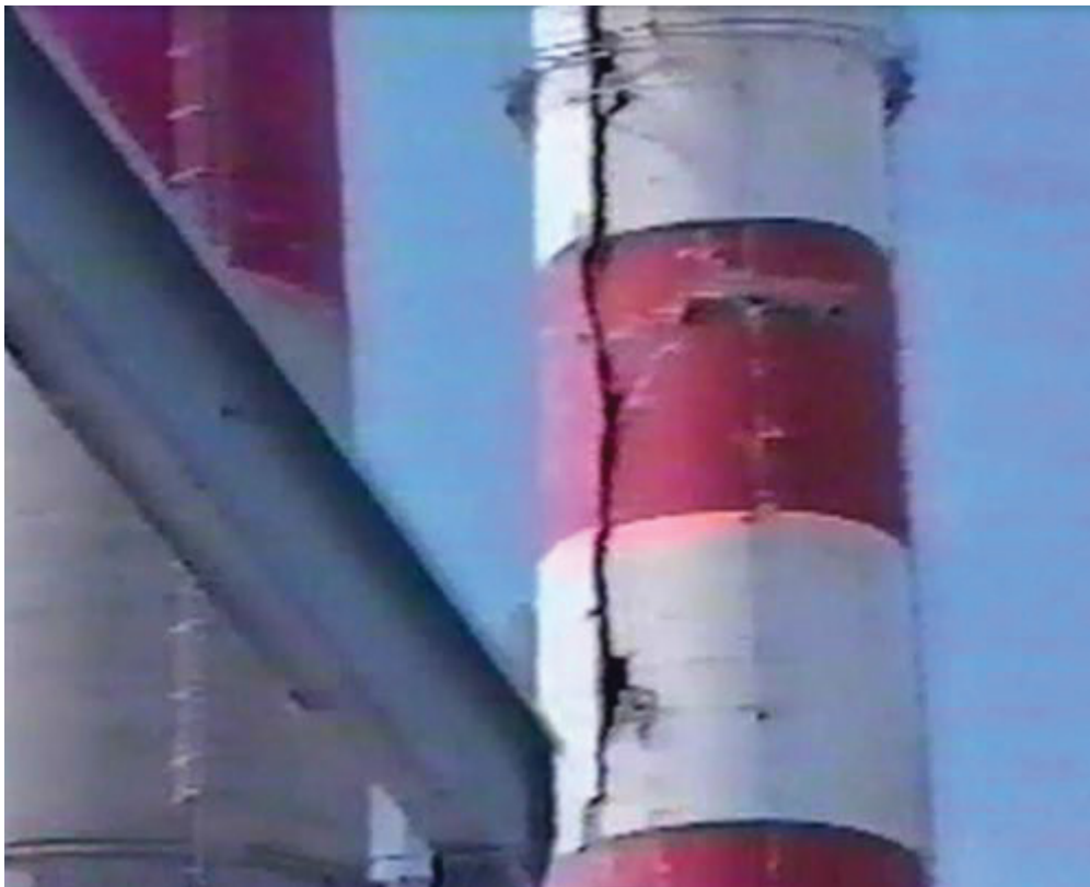
Figure 1. Structural damage to Turkey Point Unit 1 exhaust stack. (Union of Concerned Scientists 2011).
