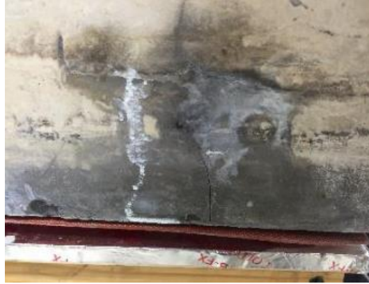
Figure 6. Damage Location 3: cracking and powder effluence.
