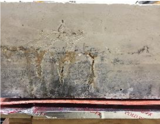
Figure 5. Damage Location 2: clear gel effluence.
