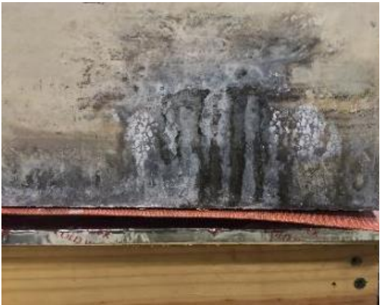
Figure 4. Damage Location 1: cracking and powder effluence.
