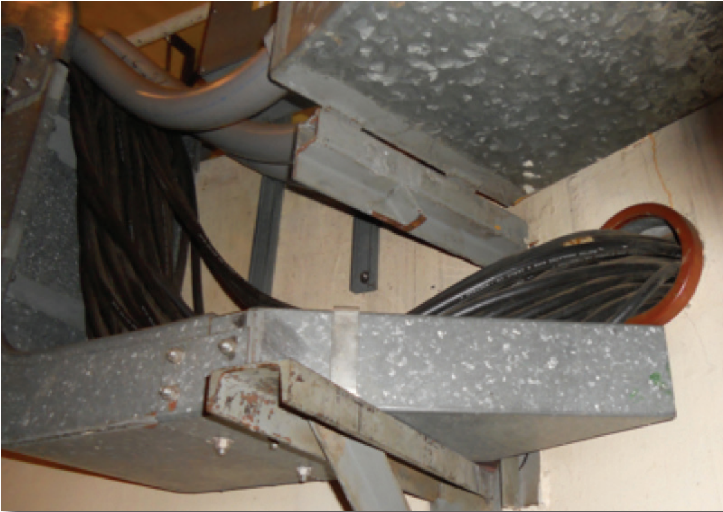
Cables harvested from the decommissioned Zion Nuclear Power Station will provide important test specimens
