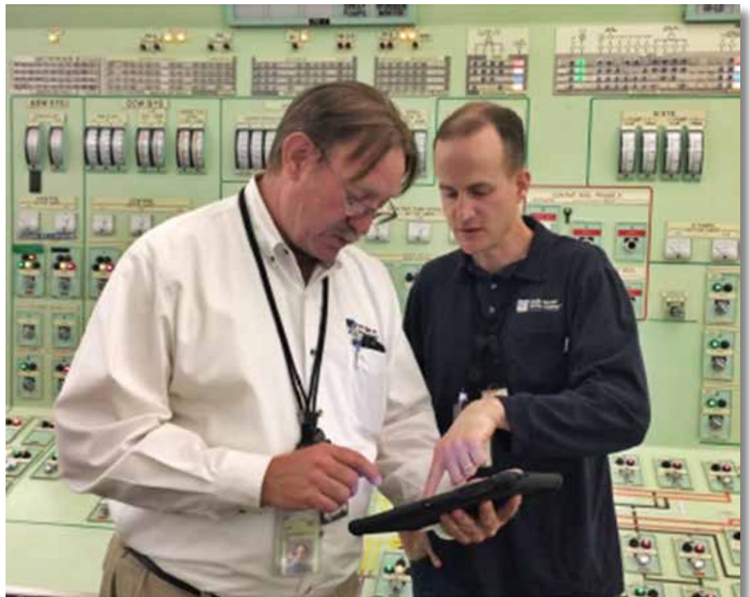
A control room operator and a field operator at Diablo Canyon Power Plant discuss a procedure using the CBP system on the handheld device.
