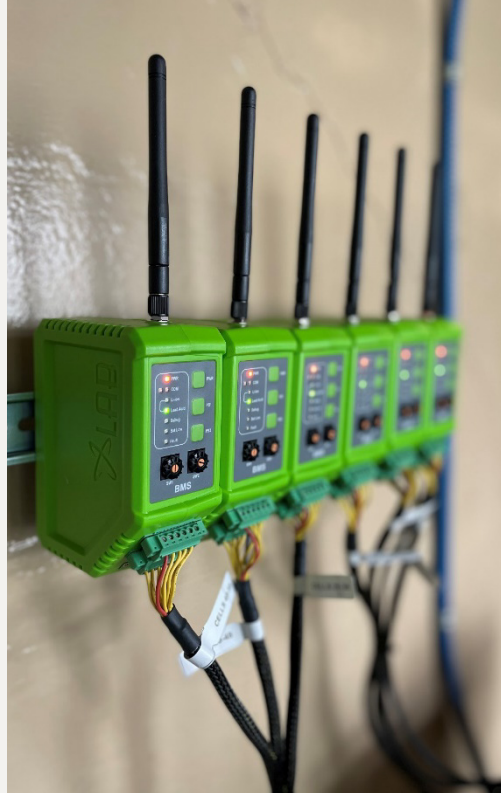
Battery Monitoring System (BMS)
