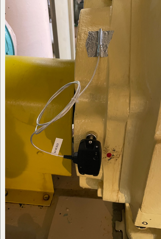
External Temperature and Vibration Sensor
