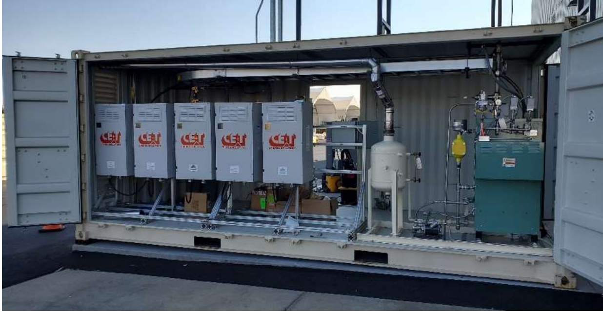
Figure 3. HTE Support Facility (used to support testing of the Bloom 100 kW e SOEC system).
