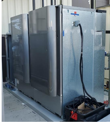
Figure 2. Photograph of a Bloom prototype 100 kW SOEC system installed at INL.
