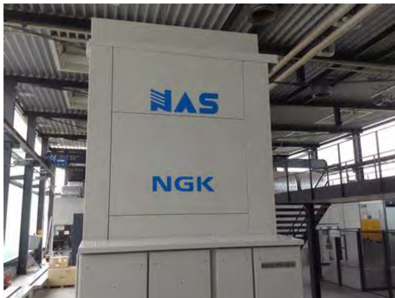
Figure C-3. Photograph of an installed NGK sodium sulfur battery module.
