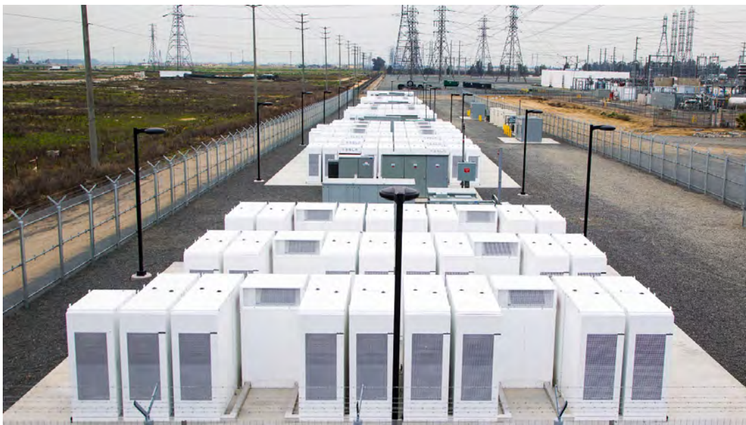
Figure C-5. Tesla 80 MWh lithium-ion battery installation in Mira Loma, CA.
