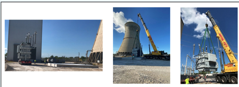
Figure 12. Installation of power switch gear for hydrogen pilot plant demonstration at the Davis-Besse Nuclear Power Plant.
