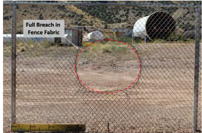
Figure 6. Explosive damage to fence.
